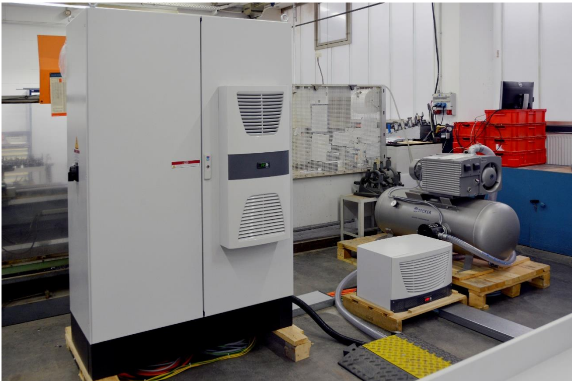
Control cabinet, recooling unit, vacuum pump with compressed air tank.
